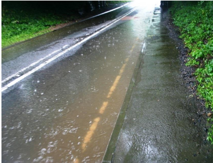
Figure 57: Surface distress associated with flooding during heavy rain.
