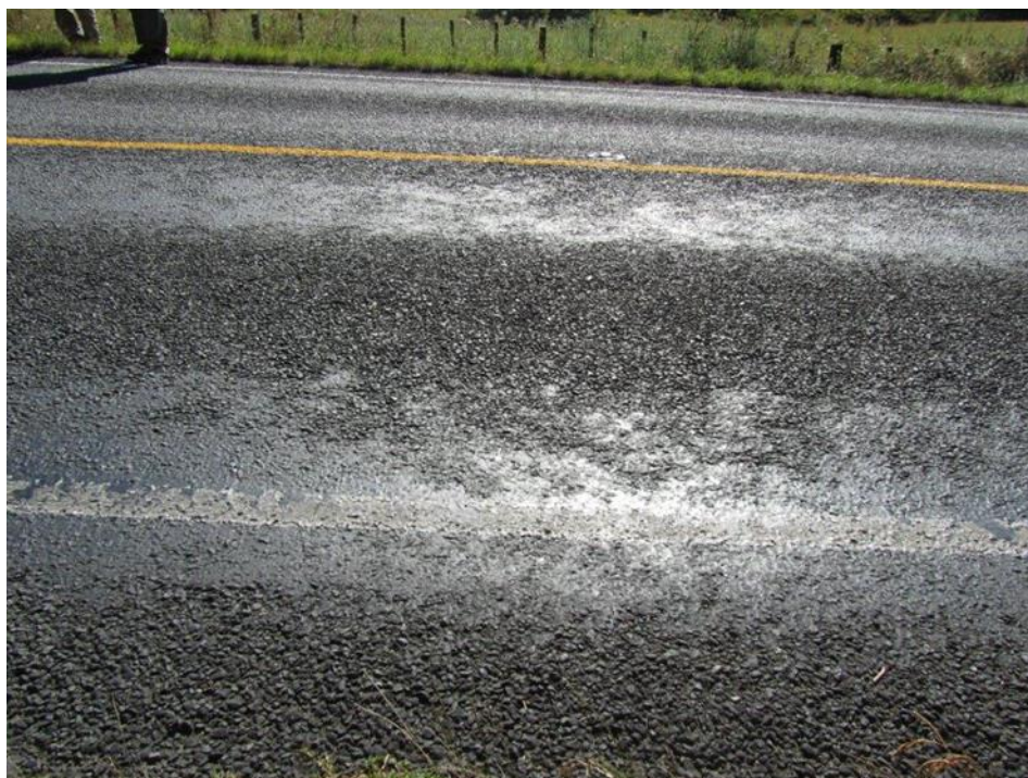
Figure 5: Typical condition of a deteriorated road surface deferred by the RAPT
