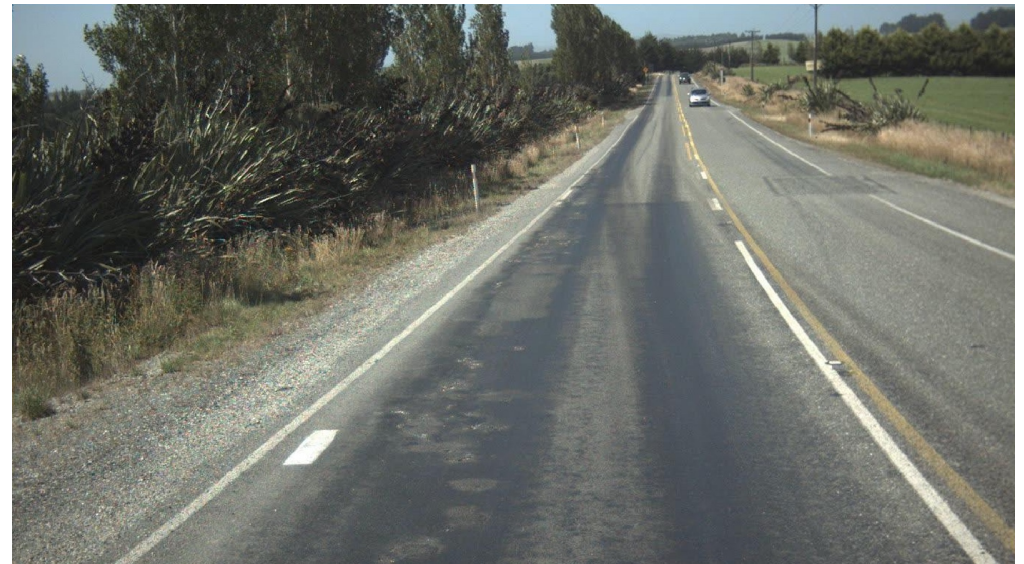
The surface in each direction on SH96 is deteriorating at different rates
