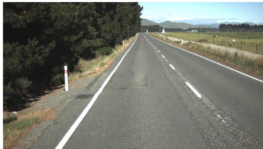
Trees on SH94 encroaching on the highway have a detrimental effect on the pavement and pose a safety risk.
