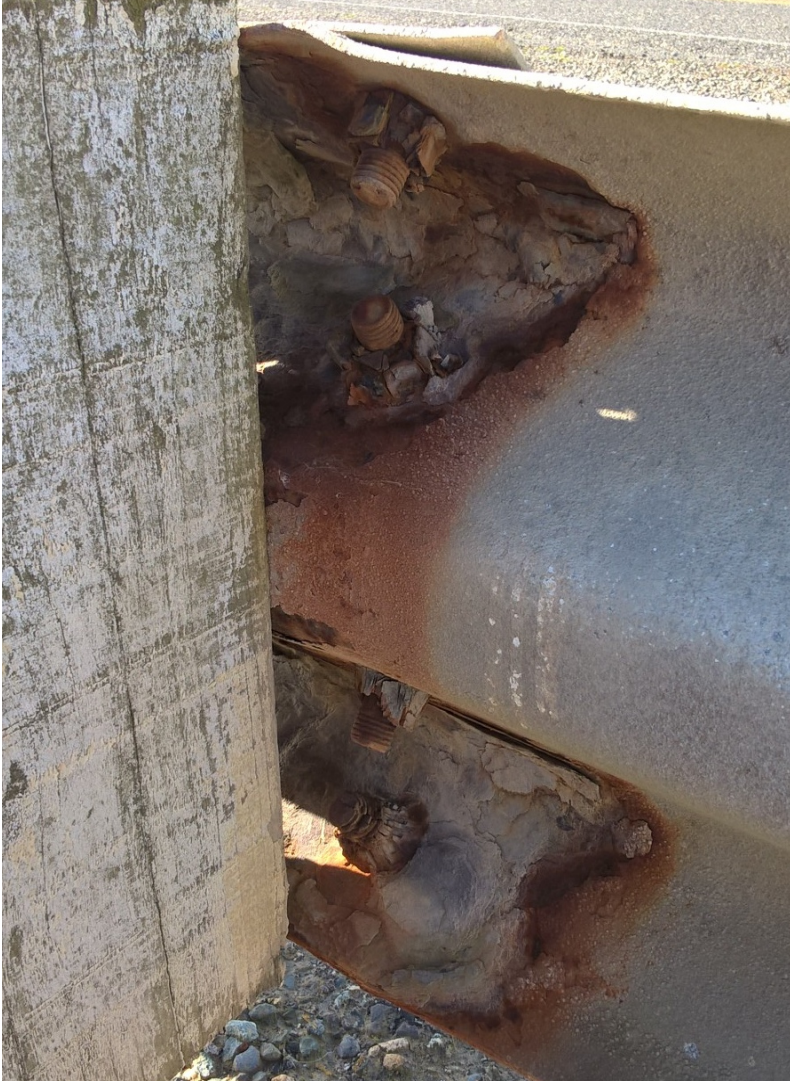
Severely corroded guardrail on SH99 requires replacement.
