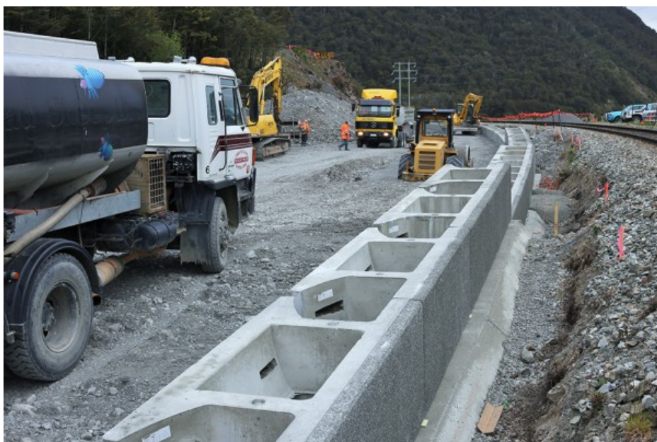
Work to realign Mingha Bluff near Arthurs Pass on State Highway 73 between Christchurch and the West Coast
