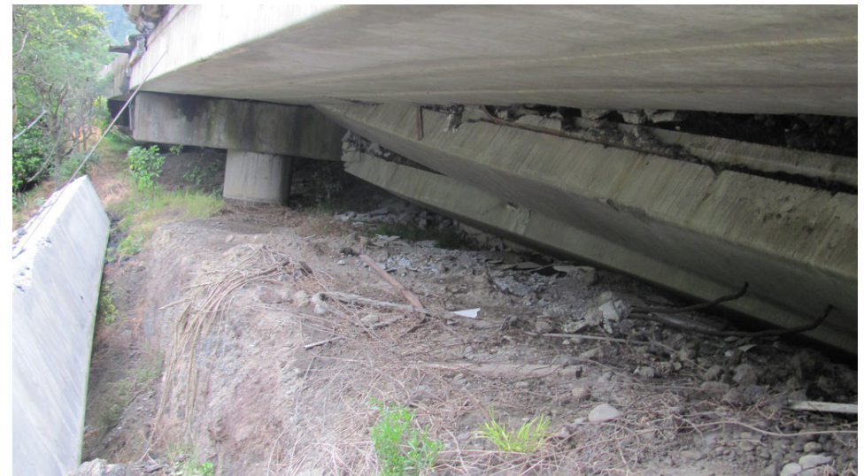
Damage to bridge that occurred in the Manawātū Gorge on 23 July 2017
