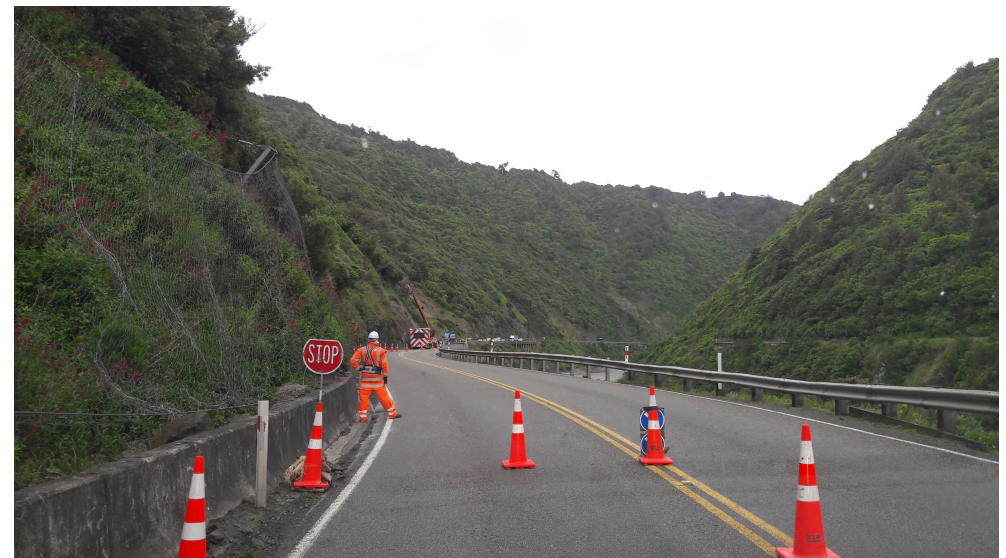
Contractors proactively removing rocks from the upper slopes of the Manawatu Gorge
