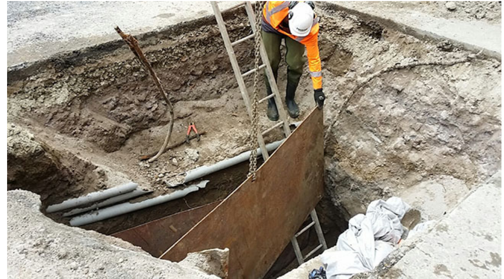
Utuhina Stream and a nearby storm water drain caused significant damage to the pavement on SH5 Rotorua in 2014/15
